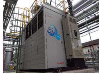
Hydrogen-fired boiler installed in Nagoya Plant
