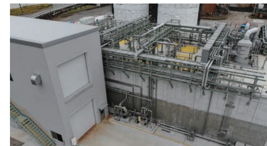
Wastewater treatment facility newly installed at the Nagoya Plant
